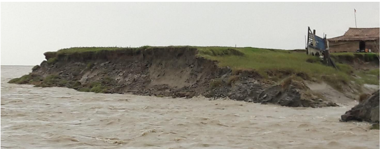
View of the western shoreline of the Gulf of Mottama, near Ah Lan Pya (29 September 2018). The steep, nearly vertical bank and the slumped blocks are evidence of the main erosional mechanism of the bank (slope collapse) that results from the ongoing landward migration of the tidal channel.
